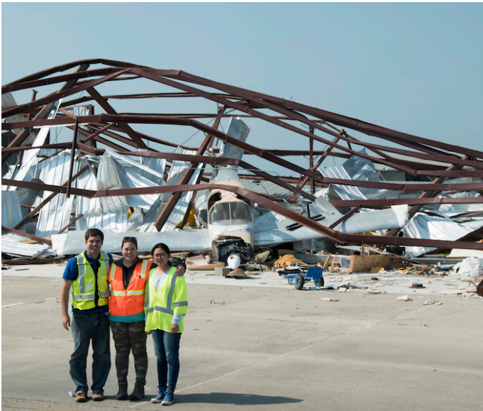
Hurricane Harvey Team 1 members (from left) Richard Wood, Kara Peterman and graduate student Yijun Liao in front of damaged hangar at Aransas County Airport (Image: Chao Sun)
