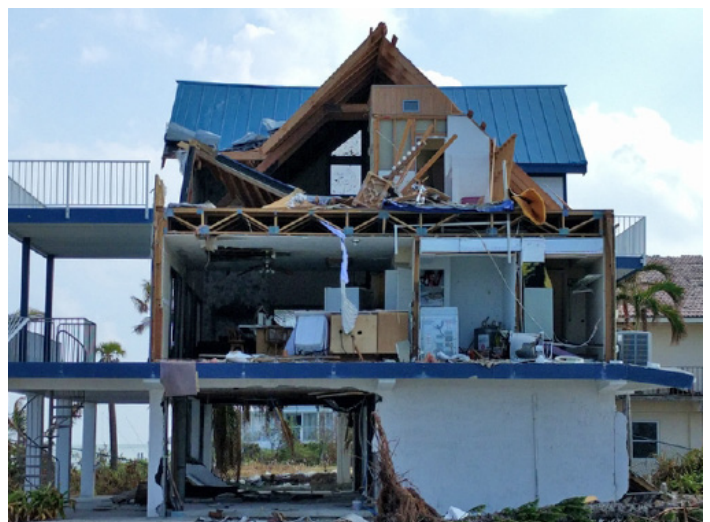
House damage in Cudjoe Key. (Image: Ioannis Zisis)
