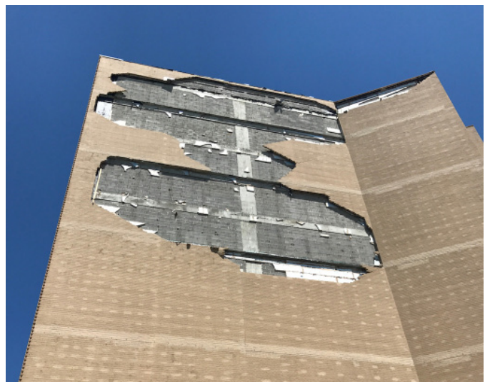
Damage to an 11-story unreinforced masonry building on Mustang Island, a barrier island on the Texas coast. (Image: Kara Peterman)
