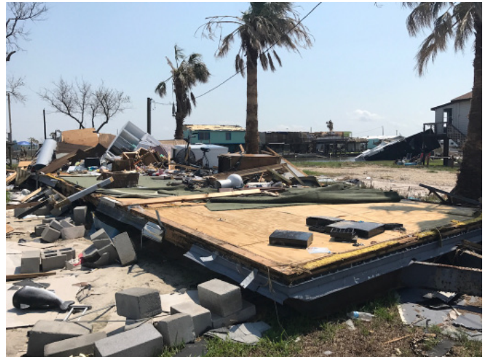
A collapsed and destroyed mobile home in Rattlesnake Point, Rockport, Texas. (Image: Kara Peterman)
