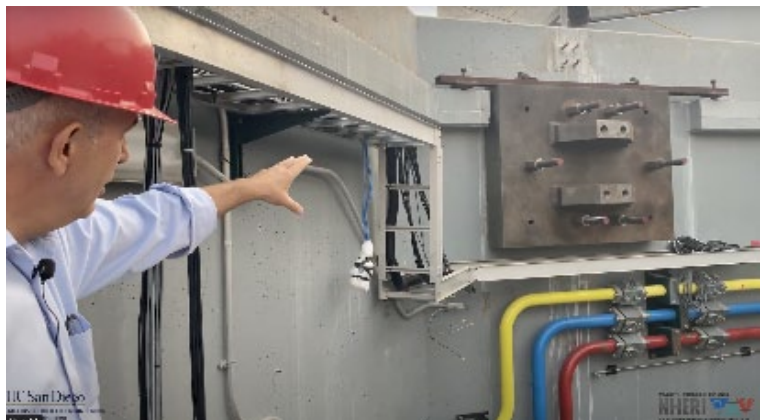
One of the steel plates to which the horizontal actuator will be anchored, shown prior to grouting.
