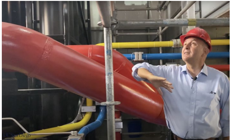
New pressure pipes have a 12-inch inside diameter, with a 1.25-inch thickness.
