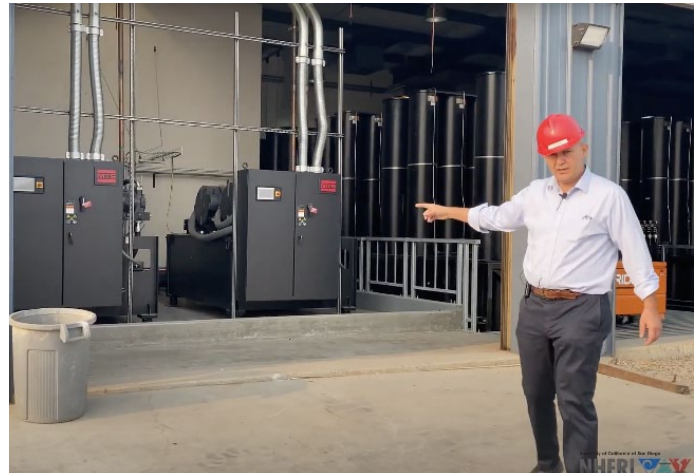
Two new pumps add to the existing two. In total, three pumps will pressurize the accumulator bank.
