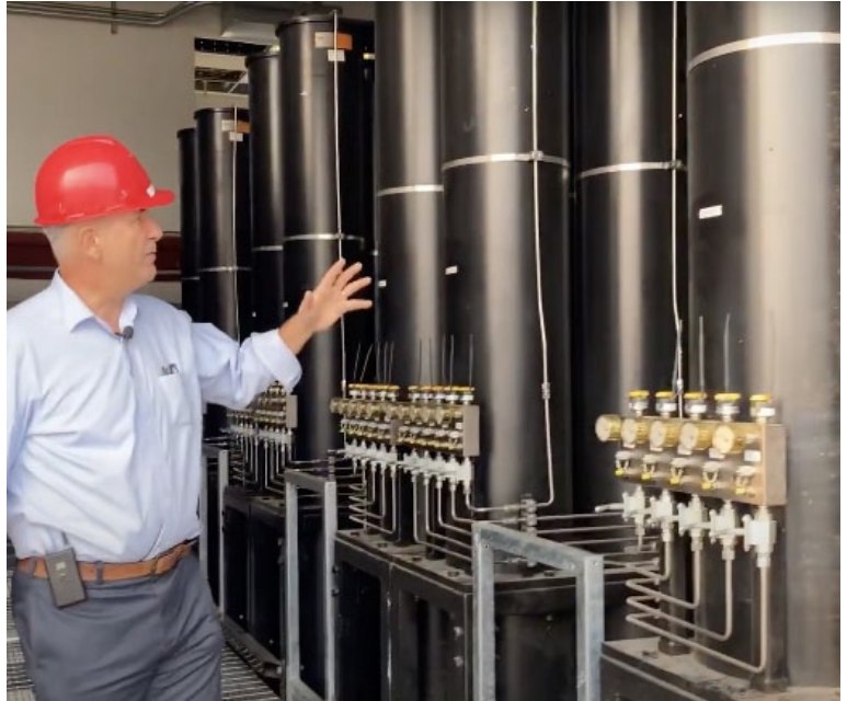
The new accumulator bank consists of 75 bottles, with capacity for 10,000 gallons of hydraulic fluid. These pressurized tanks will control the horizontal and vertical actuators that will reproduce multidimensional earthquake motions.
