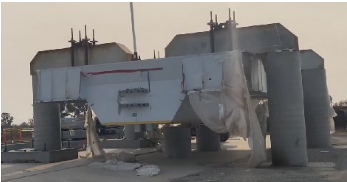
The shake table platen is being stored temporarily on reinforced concrete columns. The 145-ton platen will be machined underneath to accommodate new wear-plates and new vertical actuators.
